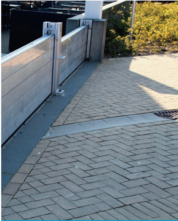
Abb. 53: mobile Flutmauer; Quelle: Embeki / stock.adobe.com
